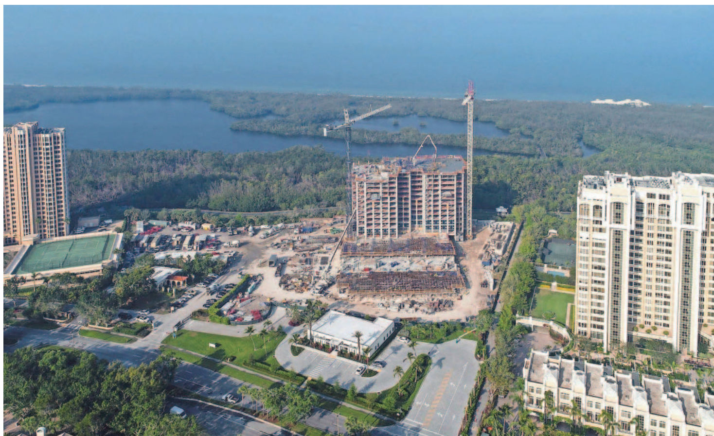
Construction continues to progress as Mystique's 15th floor has been formed and poured, and work is in progress on forming the 16th floor and supporting structural elements. CONTRIBUTED
